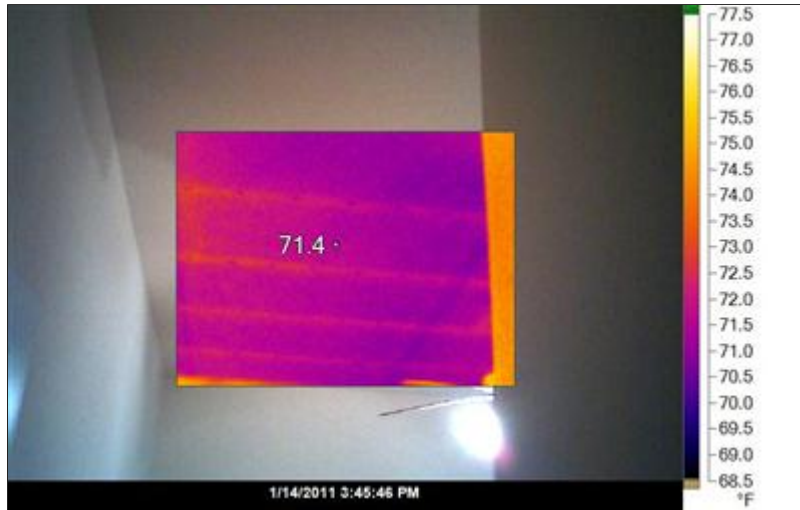
D. Picture 3 Infrared Imaging shows no insulation
