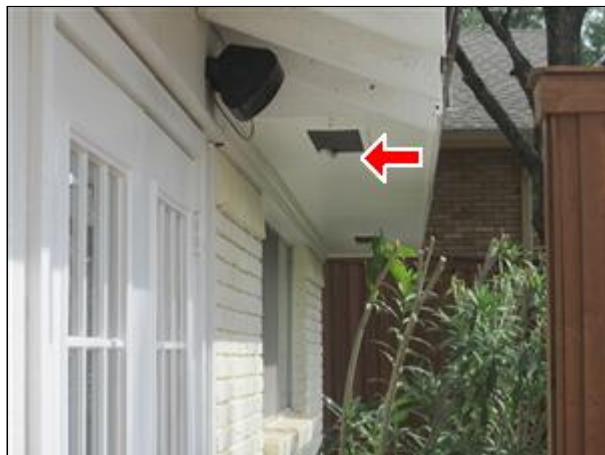
C. Picture 7 Pan drain termination point improper
