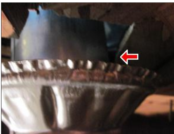
C. Picture 9 Flue close to combustibles
