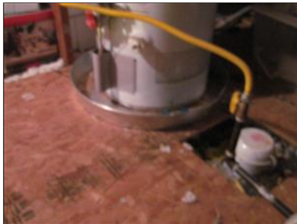
C. Picture 5 Unit not properly supported for attic installation
