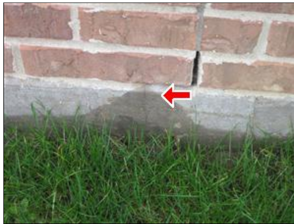
A. Picture 5 Suspected moisture from shower leak.
